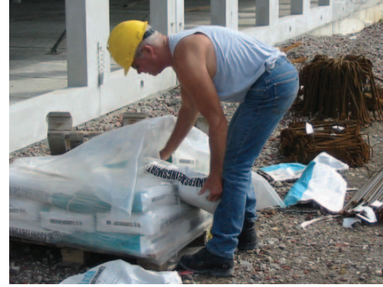
Construction worker at risk
